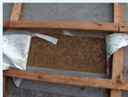
Fig. 30: Mould infestation underneath a microporous underlay membrane – the wood fibreboard underneath the membrane has become damp due to weak passive moisture transport, thus providing favourable conditions for mould growth.
