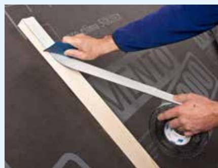
Fig. 6: Sealing of perforations around counter batten fasteners with nail-sealing tapes/ compounds or through the verified self-sealing capacity of the membrane itself.
