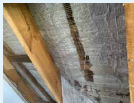
Fig. 12: Old, damaged underlay membrane (with scrim reinforcement) – outgassing of volatile plasticisers has led to significant embrittlement.
